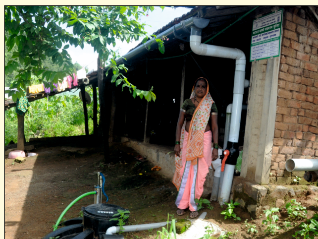
Rain Water Harvesting
